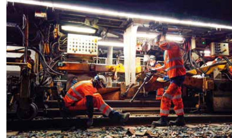
The NGE BOA factory train can replace and upgrade 270 km of track per year
