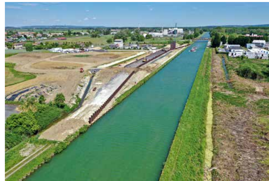
NGE delivered the first quay areas of the future Seine-Nord Europe Canal in 2022
