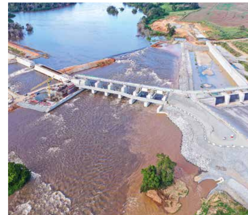
Work on the Nachtigal dam in Cameroon was 80% complete by the end of 2022
